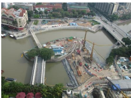
Figures 6-10. Progress photos of river diversion in order to create a jobsite.
