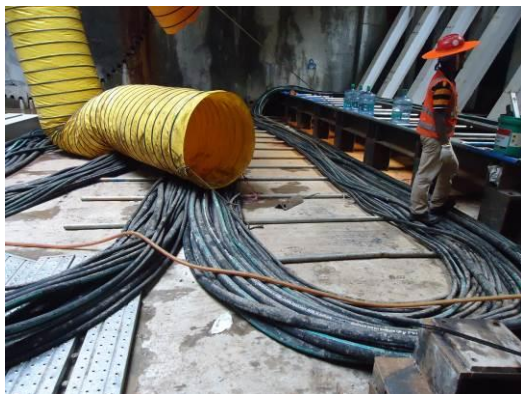
Figure 13. Umbilical hoses in shaft bottom.
