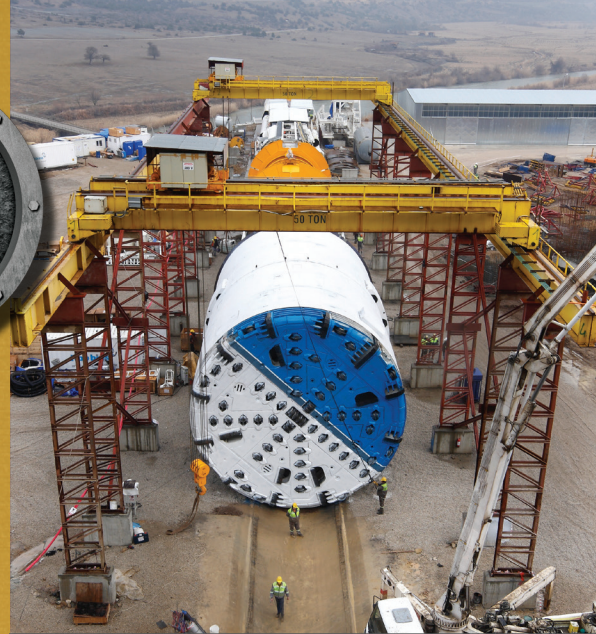
Onsite First Time Assembly of a 10.0m diameter Double Shield TBM in Turkey
