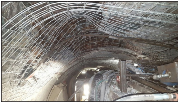
Figure 13. 8th December 2015, McNally System as additional support due to material detachment
