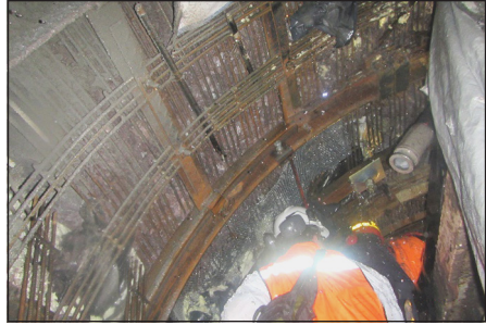
Figure 15. Initial support including McNally slats and water inflow conditions
