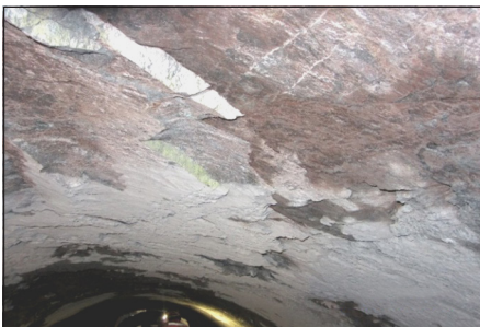
Figure 5. Planar roof and sub-horizontal joints
