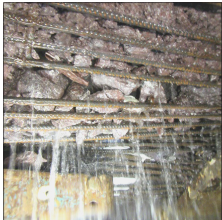
Figure 16. Initial support including McNally slats and water inflow conditions
