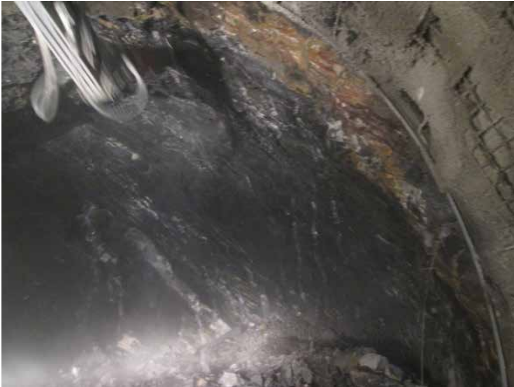
Figure 7. General view of tunnel face in the risky area for TBM. Note high water inflows.
