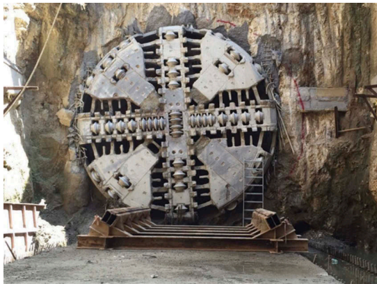
Figure 9. Condition of the new cutterhead after breakthrough into the final receiving shaft.
