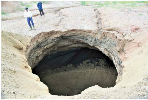
Figure 7. Sinkhole above the machine.
