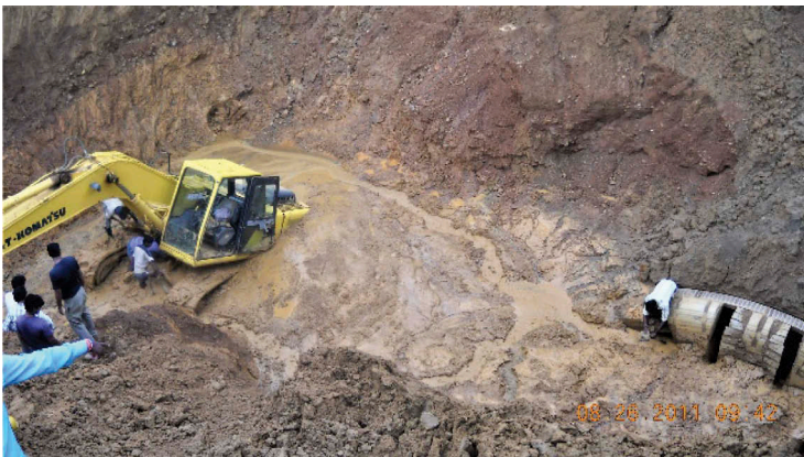
Figure 6. Liquefaction of the soils.
