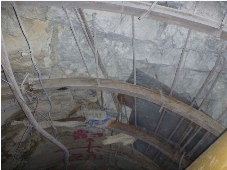
Figure 3. Example of inappropriate rock support.
