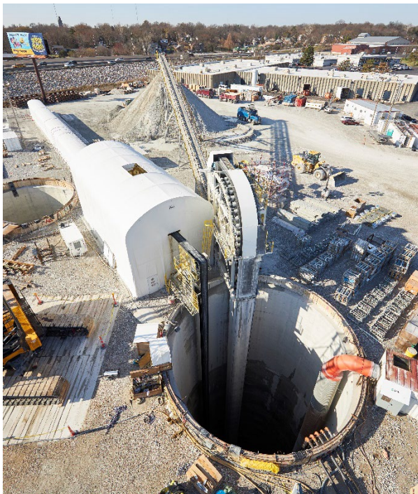
Figure 9. The Deer Creek shaft and continuous conveyor system
