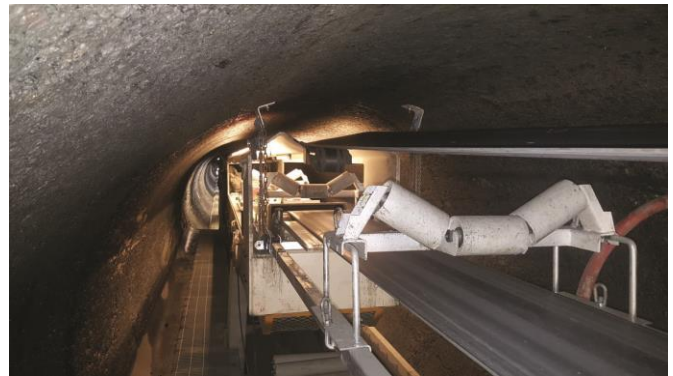
Figure 9. Crown-mounted conveyor at Salvasskardelva
