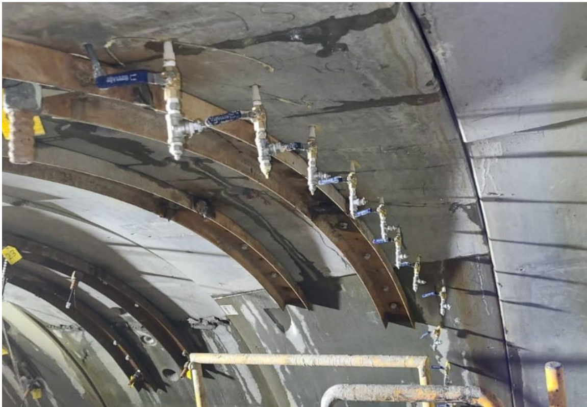
Figure 13. Chemical grout collar radial injection ports to stabilize ring along with steel channel.
