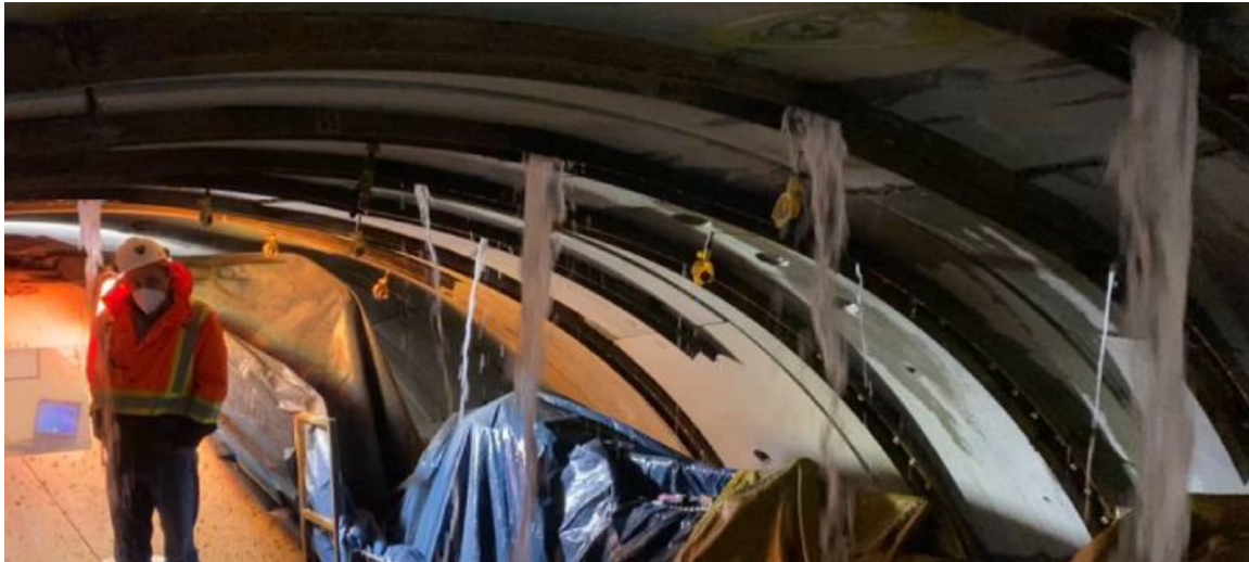
Figure 12. Significant, sustained water inflows from the rock formation above the tunnel crown (Solecki et. al., 2022).
